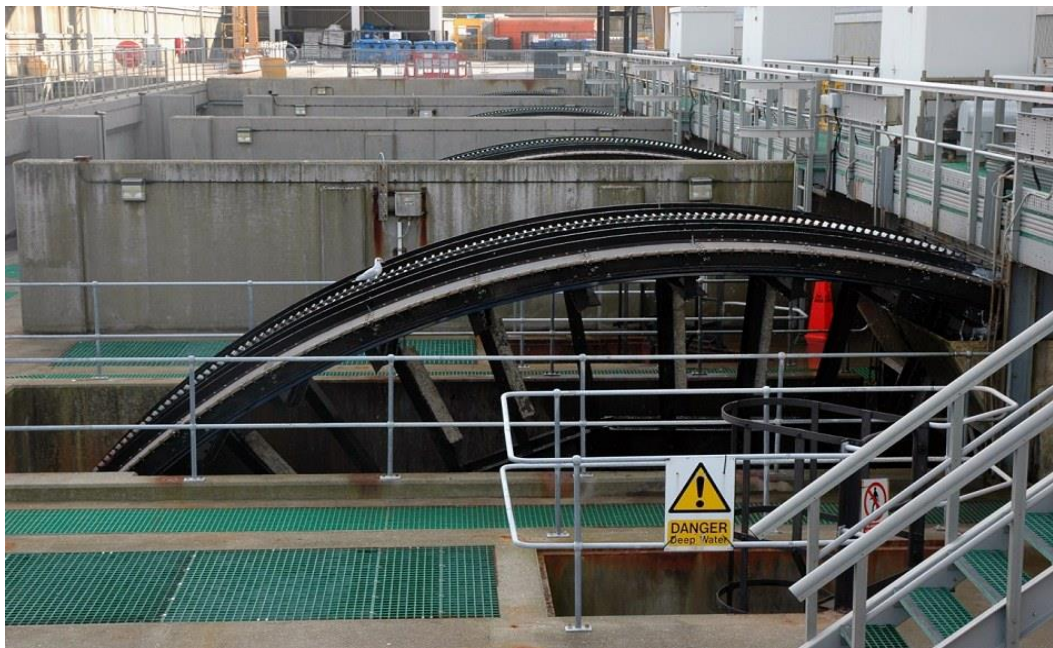
Figure 2.1 The four drum screens at Sizewell B
